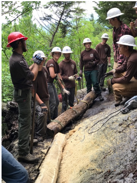
[Left: ACE crew setting a crib log on a steep rock face.]
